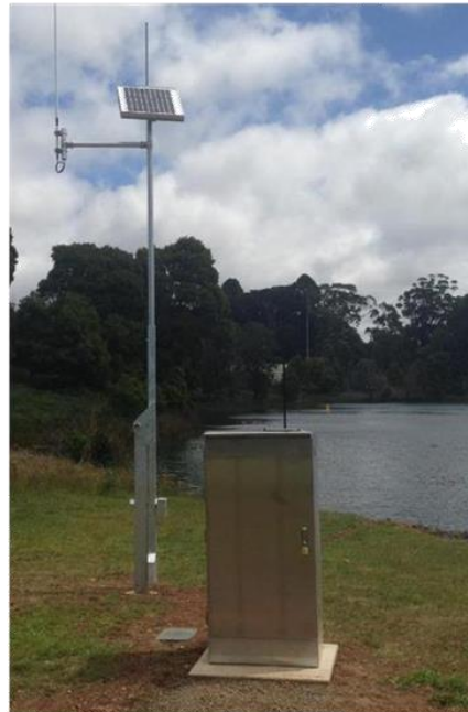
Figure 1 –Automated River Height Monitoring Station
